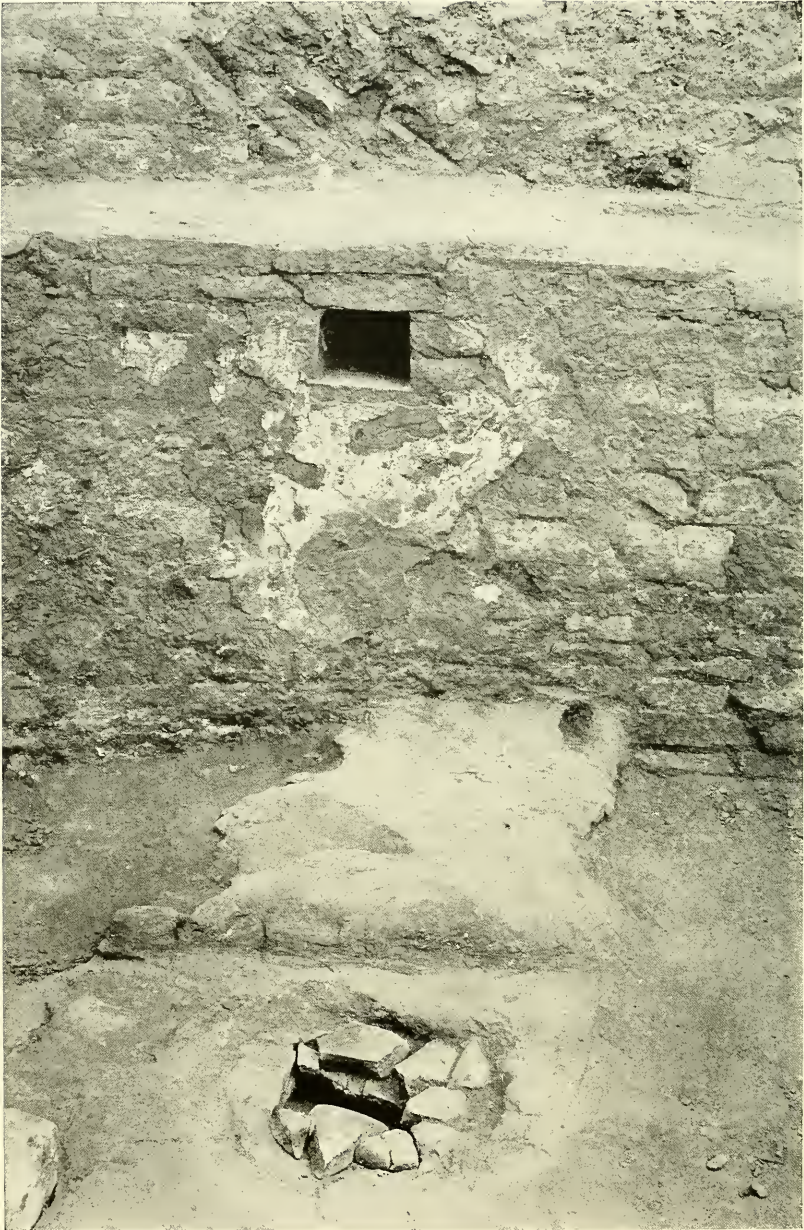
PART OF THE MAIN WALL OF KIVA I, WITH THE BUTTRESS WALL AND ITS EASTERN NICHE, THE ALTAR PLATFORM, AND THE SHÍPAPULIMA
